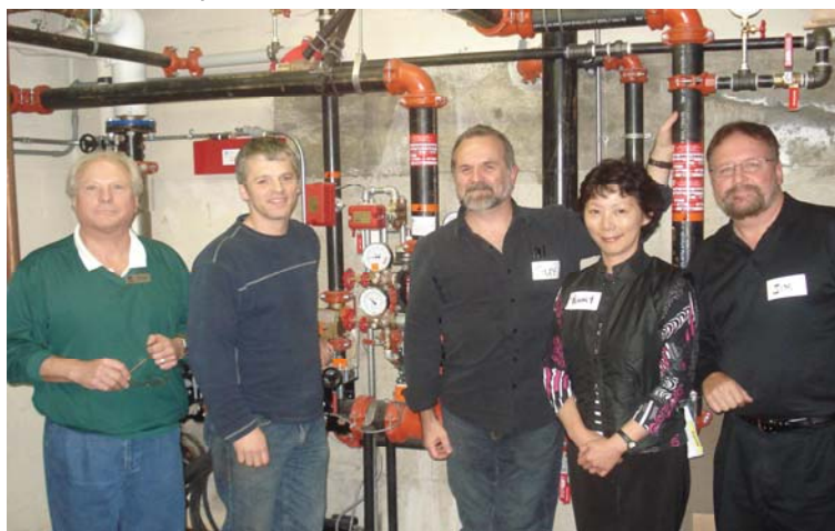
From L to R: Tom Nowak and Michael Bryant of L'Arche, Guy Clarkson (Gisborne), Penny Lim of L'Arche and Jim Sawers (Gisborne) in the sprinkler system control room.
